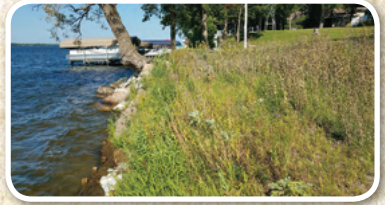
Project pictured above did not receive adequate water during Year #1.
