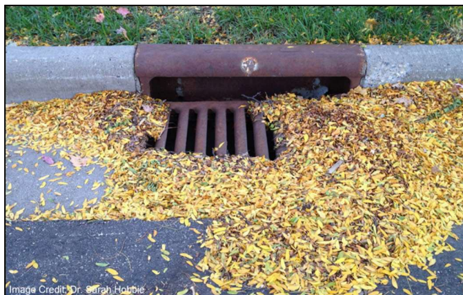
Figure 1. Leaves, seeds, and other tree debris accumulating in road gutters will eventually wash into storm drains and downstream waterbodies unless they are removed.
